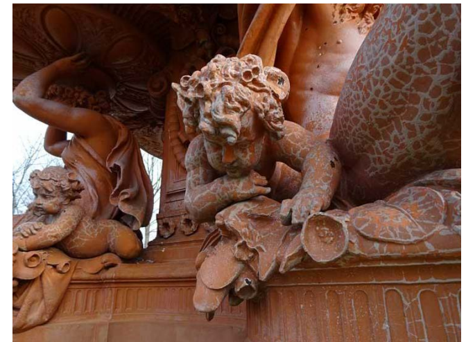
Fig 43: Current condition and signs of degradation
